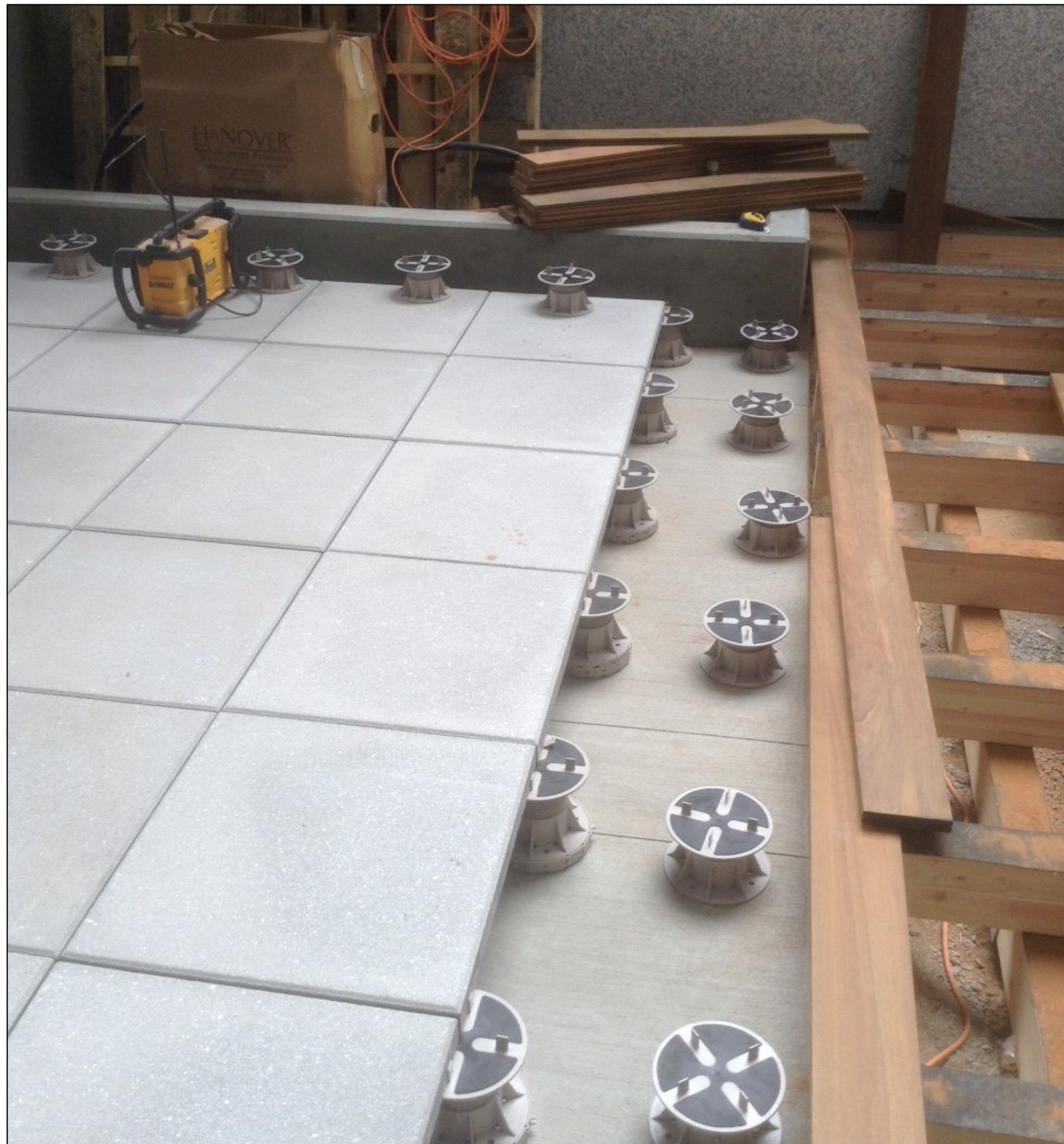
The finished floor surface is only slightly above the building's footings. An elevated paver system designed for rooftop patios, created level patio and deck space above the sloped concrete drainage system. (North Courtyard)
