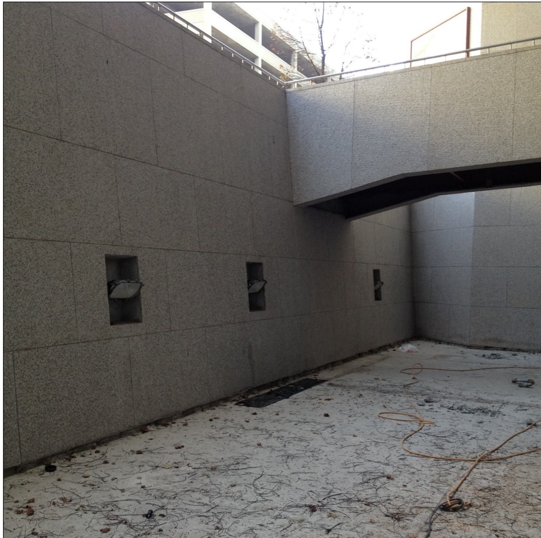
The existing areas, almost 20 feet below street level were cold, stark, and uninviting. Access was a challenge as were solid bedrock, drainage, shade and finding space for mechanical, and water storage for the two water features. (East Courtyard)
